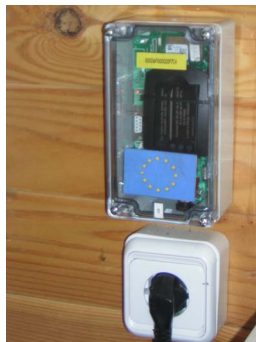
Figure 3. Node. Measurement of energy consumptions parameters and switching on/off. ZigBee communications.
